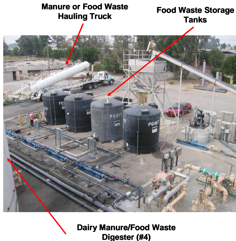
FIGURE 4-1 Manure and Food Waste Co-Digestion Facility at RP-1
