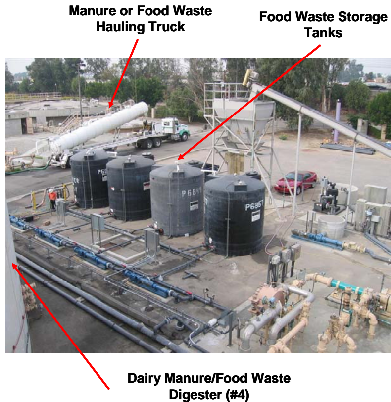
FIGURE 4-1 Manure and Food Waste Co-Digestion Facility at RP-1
