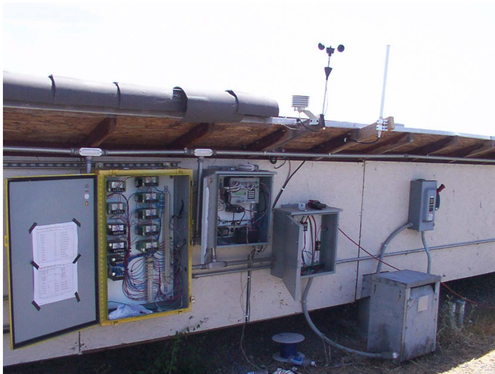
Figure 3. Datalogger and Transducer Enclosures
